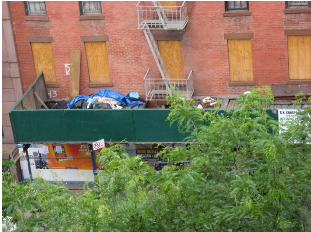
Early August 2009: Presence of garbage and suitcase on scaffolding
