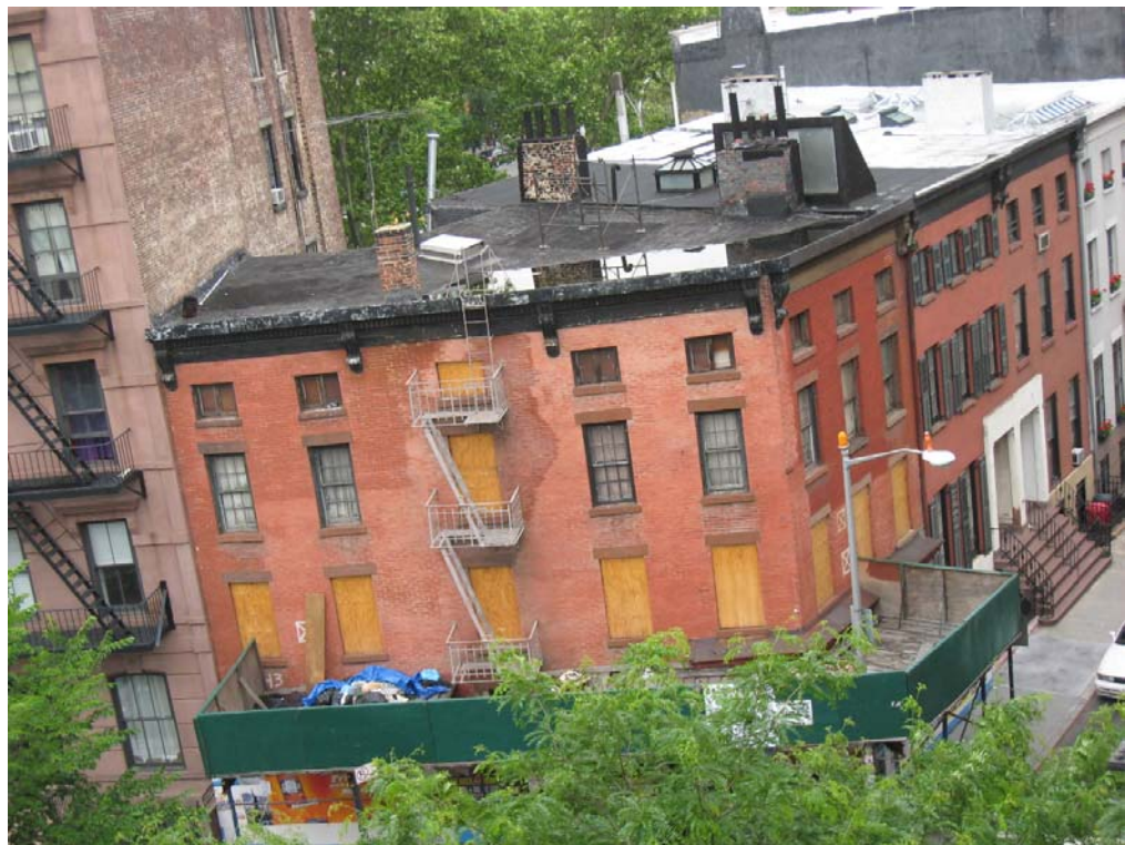
Early August 2009: Water pool on roof visibly warping brick facade
